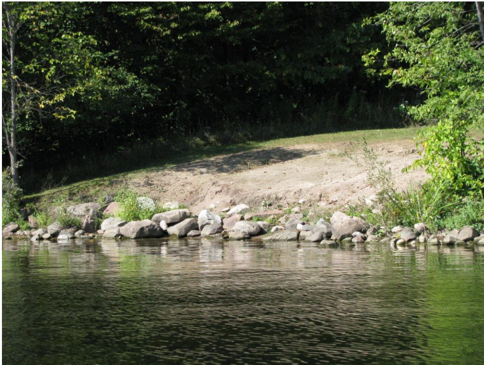
Erosion of sandy soils along the shoreline of Crowe's Line Beach (North shore of Pigeon Lake, September 2015)
