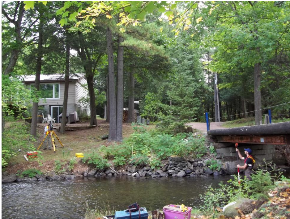
Kawartha Conservation staff installing water flow monitoring equipment near the outlet of Nogies Creek (Bobcaygeon, September 2012)
